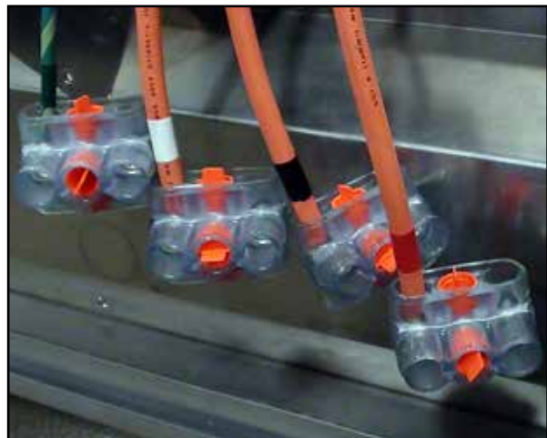
Figure 10: Power Entrance Box
