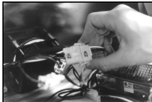
Figure 13: Disconnection of LED Module Panel Power Cable
