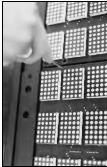
Figure 22: Loosening of 1/4-Turn Fasteners (1.2" & 2.1")
